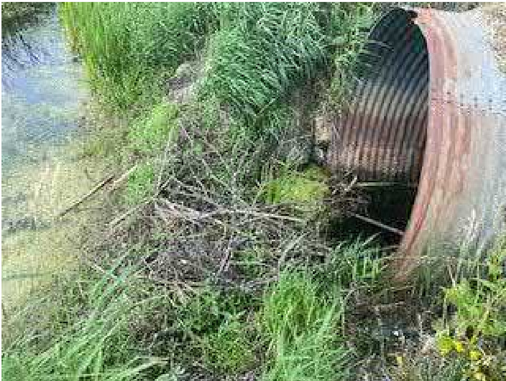
Photo 8: Debris at Culvert Downstream Invert Out Dated: 06/29/2021
