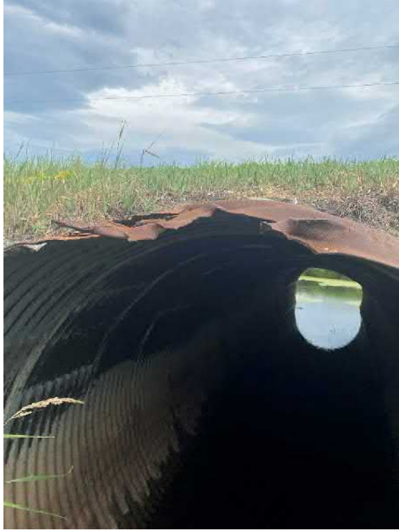
Photo 5: Culvert Outlet Corrosion Dated: 06/29/2021
